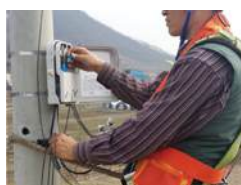
Work Belt on the telephone pole
